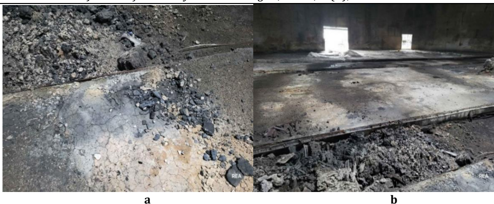
Fig. 1. Image of the consequences of the fire in the agricultural premises as a result of the explosion: a – fire epicenter; b – floor and walls around the epicenter
