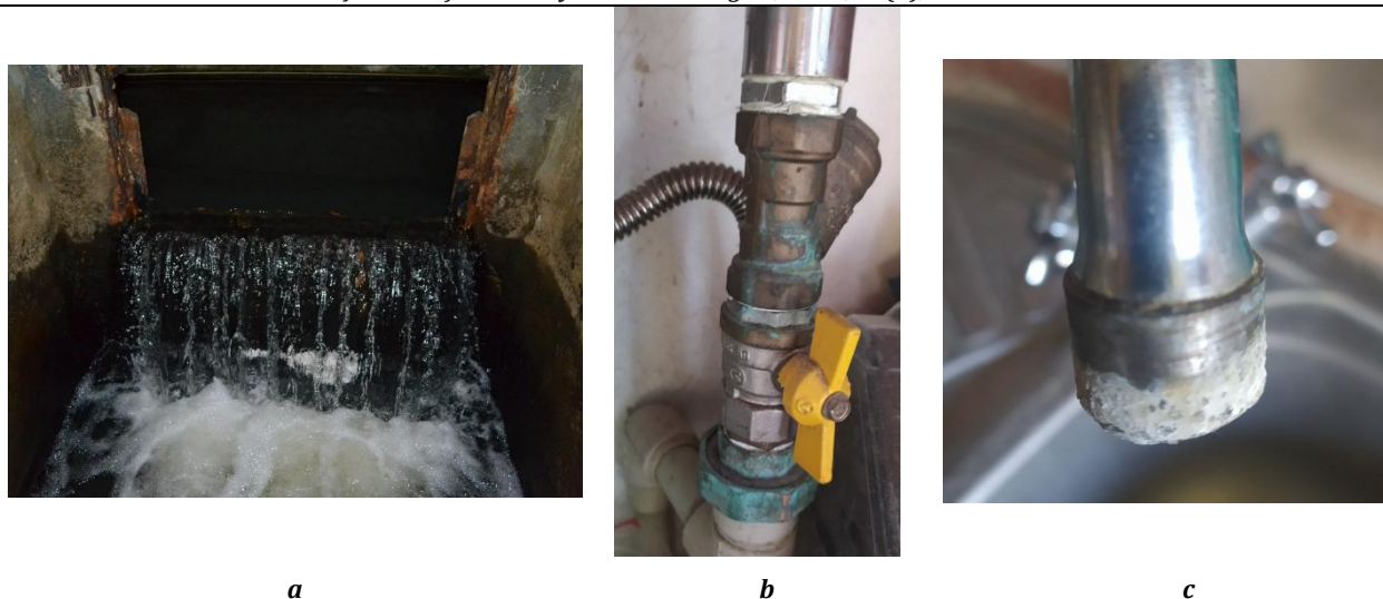
Fig. 3. Examples of corrosion during water transportation: (a) corrosion of equipment at a water treatment station; (b) corrosion of faucets in centralized water supply; (c) corrosion of faucets in centralized water supply
